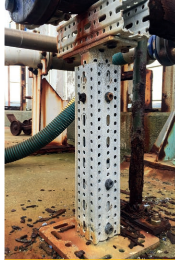
... after 6 years of weathering
